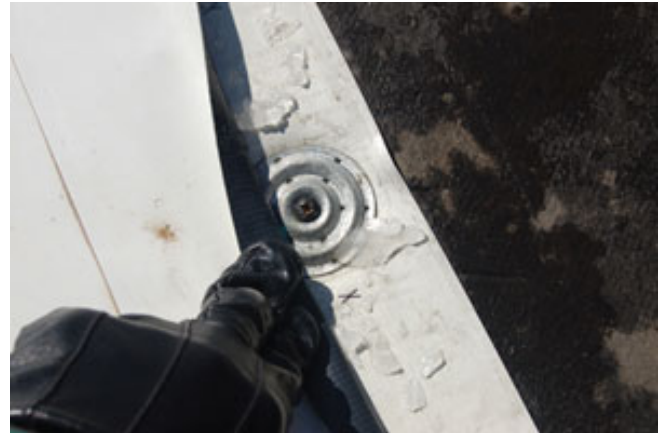
Photo 2: Ice accumulation up to 1/2 of an inch thick has been observed in laps.
