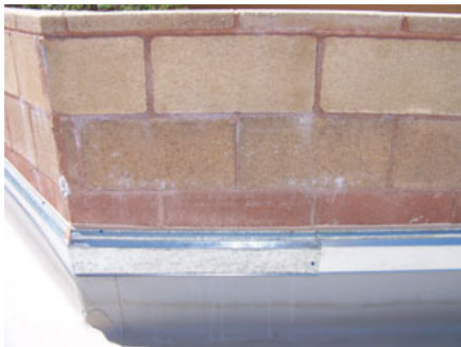
Photo 3: This masonry wall expanded so much the control joints squeezed shut and mortar debonded, resulting in moisture intrusion and deterioration.
